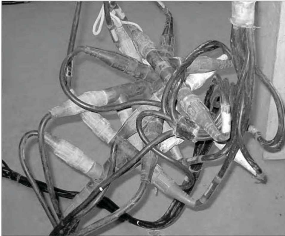
Figure 66-8 Unsafe condition of ganging tees together
